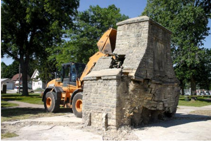
A Kasson city employee tipped over the top half of the fireplace chimney in Veterans Memorial Park Wednesday. The fireplace was removed to make way for a new 40' x 80' park shelter.
