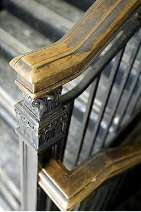
A stairway in the former Kasson Elementary School, which has been named one of Minnesota's top 10 most endangered historic places.
